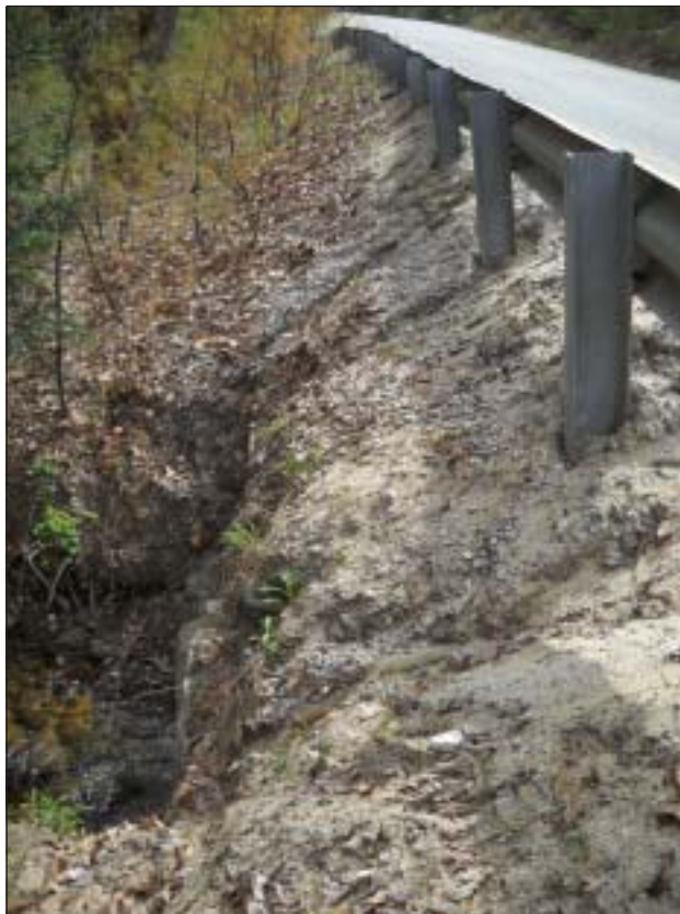
Forrest Edwards Road site before erosion control work.
