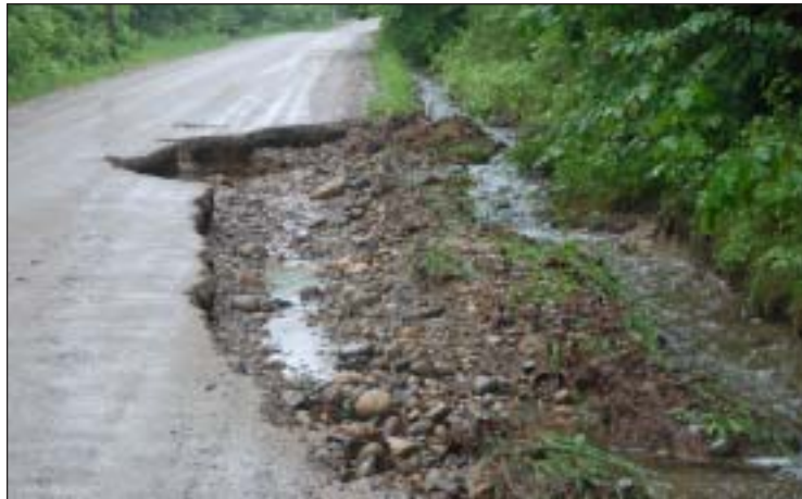
Cobb Hill Road, Otisfield, after the June 2-3 rains. (Photo Bob Tracy)
