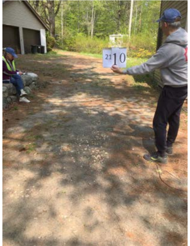
Site 21-10: Low impact driveway site that has identified sheet erosion.
