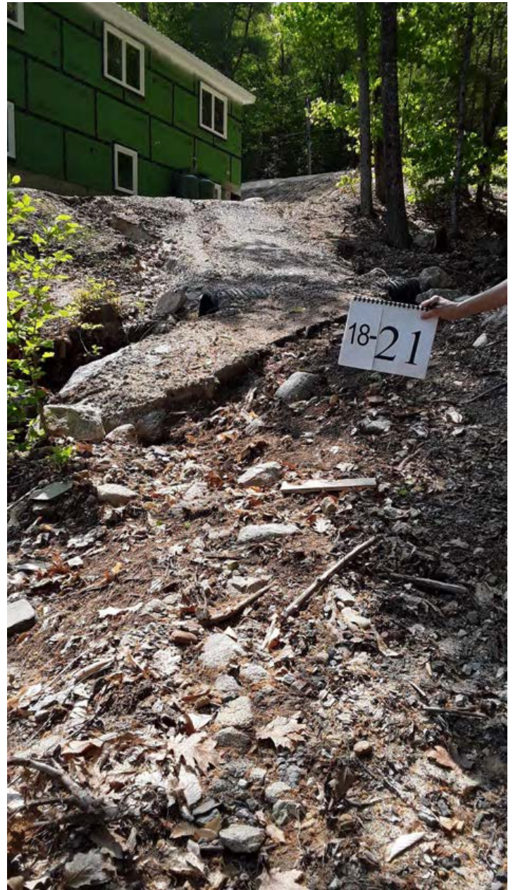
Site 18-21: High impact residential site. Few erosion and sediment controls for active construction on site.
