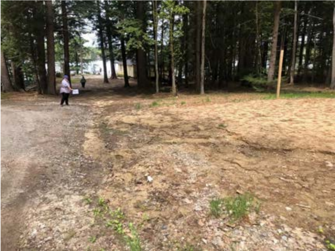
Site 7-03: A medium impact 'other' site that has identified gully sheet erosion at a volleyball court in Sector 7
