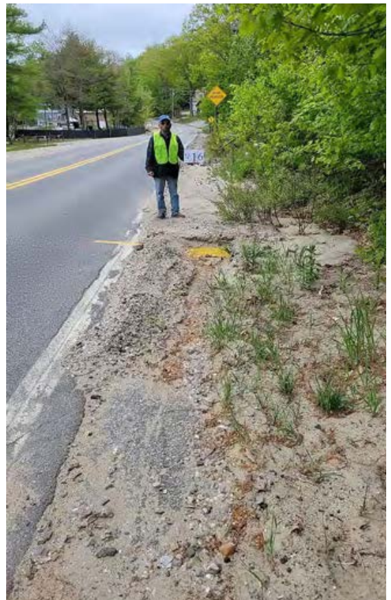
Site 12-16: High impact state road site that has identified gully surface erosion, a clogged and unstable culvert, ditch erosion, road shoulder erosion, and buildup of winter sand, and evidence of a considerable amount of sediment and gravel washing into a catch basin.
